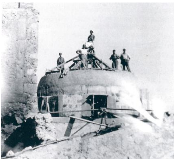
Fig. 02 - San Pietro Infine (CE), the post-war reconstruction of the dome of San Michele Arcangelo with the use of reinforced concrete (Zambardi 2003)
